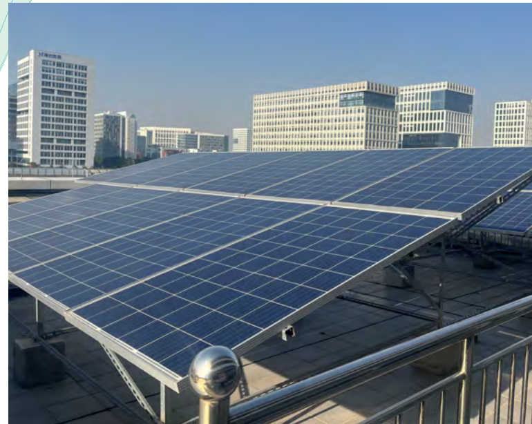
Suzhou, China facility solar panels.
